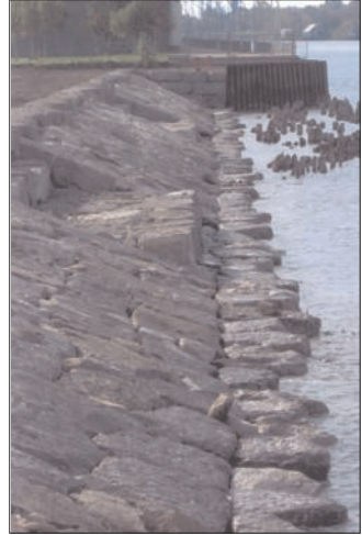
After renovation. Minimal damage to wharf piers with stairway access to water
