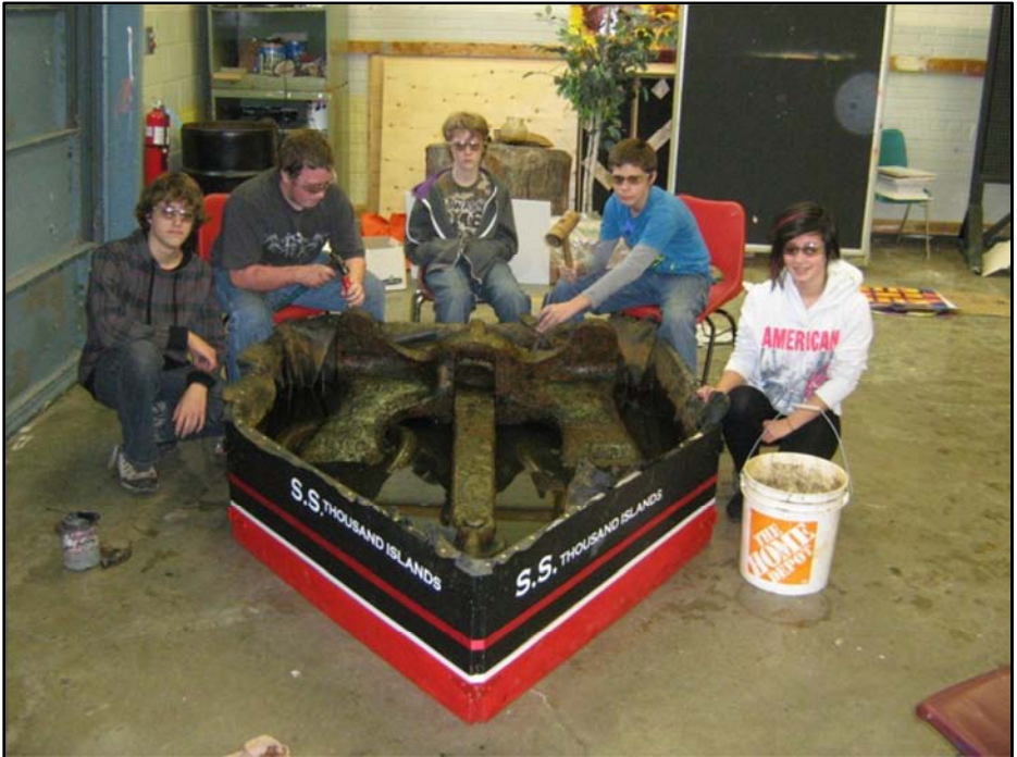
Students removing the corrosion layer with hand tools. From left: Theo Schaefer Scovil, Chris Lautsch, Ken Wardle, Troy Sargent, and Natasha Carr. (TISS)
